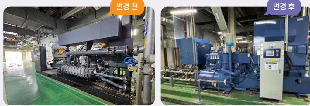
Utility Turbo Compressor
